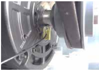
The BPK-IM2 was selected due to limited space. Installation was finished within 15 minutes.
