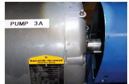
Hot Water Recirculating Pump
