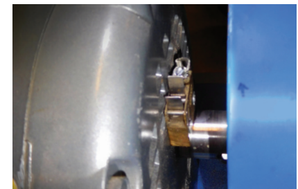
BPK-4 on Pump Motor
